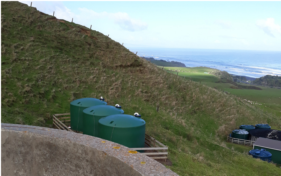
MOKAU WATER SUPPLY - NEW STORAGE TANKS
